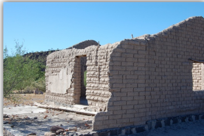
Deteriorating adobe building in San Ignacio, Baja California, with plastered cement on the outside walls.
